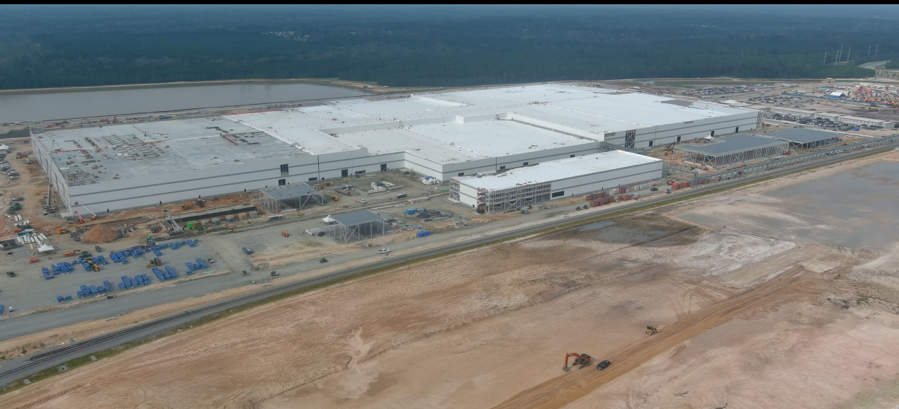
LGES-Hyundai Motor - HMC JV EV Battery Plant, Gllabell, GA 2,400,000 SF | 130 Acres | 27.5 GWH Annual Capacity | $4.3B Investment
