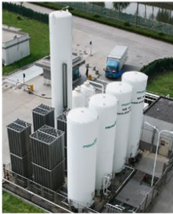
On-site gas generation
