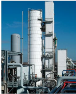
Large air separation unit and pipeline system
