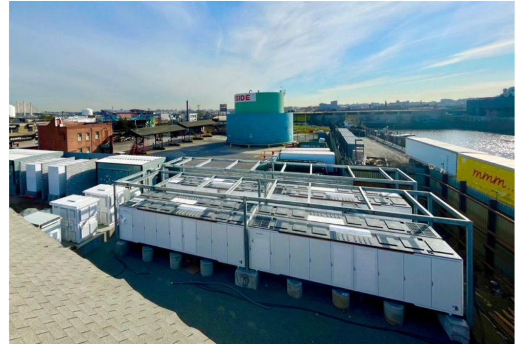
Microgrid Network (MGN) 5MW BESS, Brooklyn NYC.
