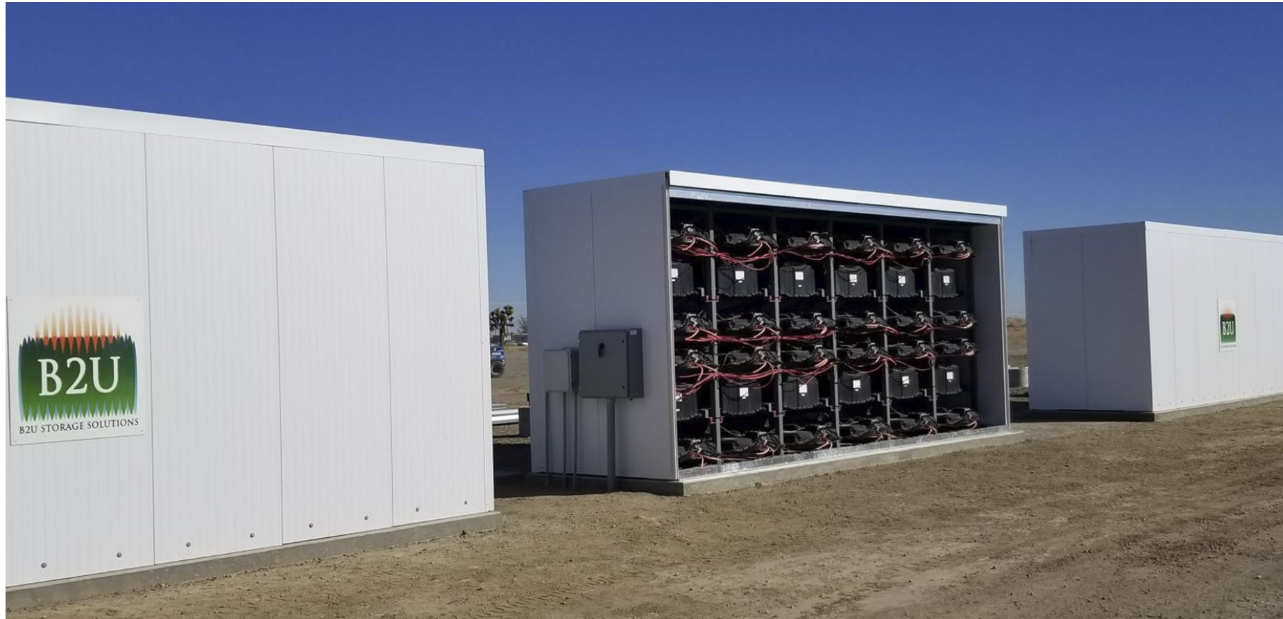
EPS Cabinet with Honda Clarity Batteries
