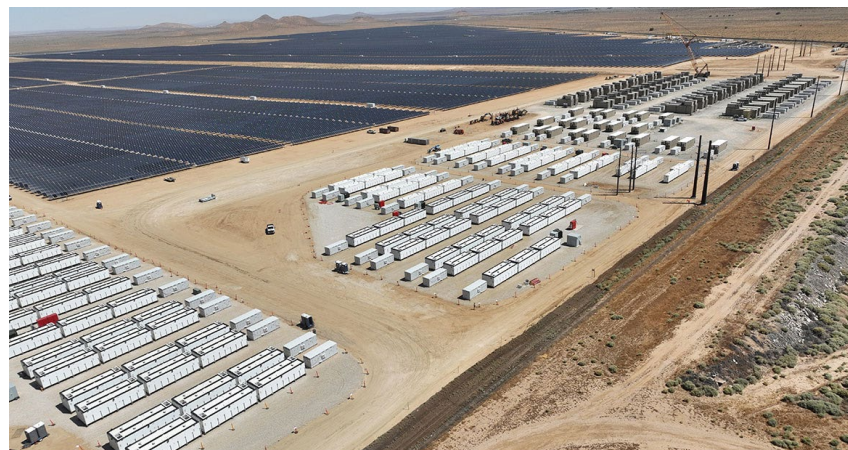
Solar PV and 3.3 GWh of battery Kern County, California
